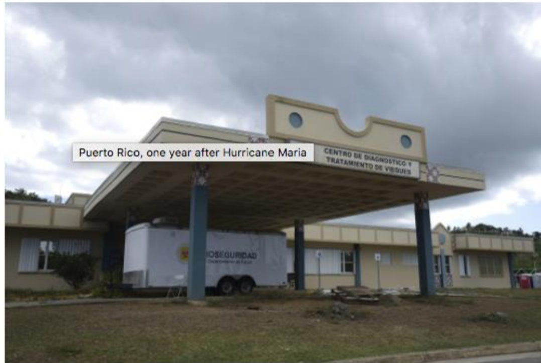
The facade of the shuttered Diagnosis and Treatment Center where dialysis patients once received treatments, in Vieques, Puerto Rico. Weeks after Hurricane Maria hit, health officials declared it contaminated and ordered that it be permanently (Carlos Giusti / AP)
